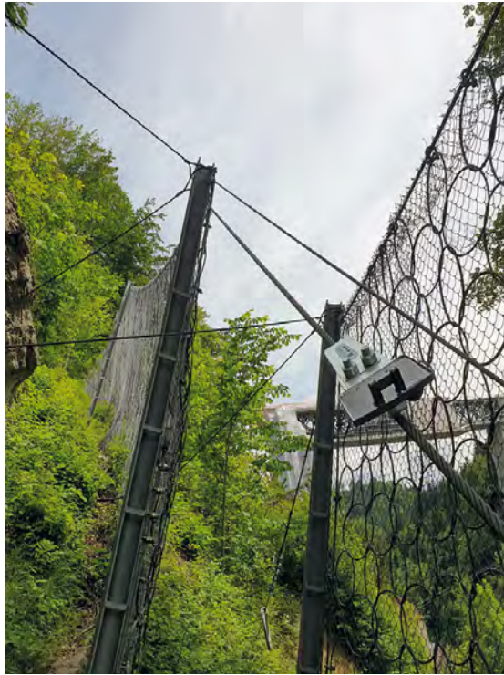
Fig. 1: Rockfall barrier with sensor device
