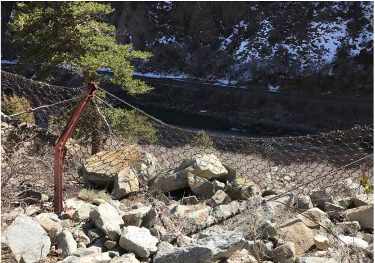
Figure 5. Rockfall barrier impact at Glenwood Canyon, CO, showing continued performance even after impact. (Photo courtesy of Colorado DOT.)
