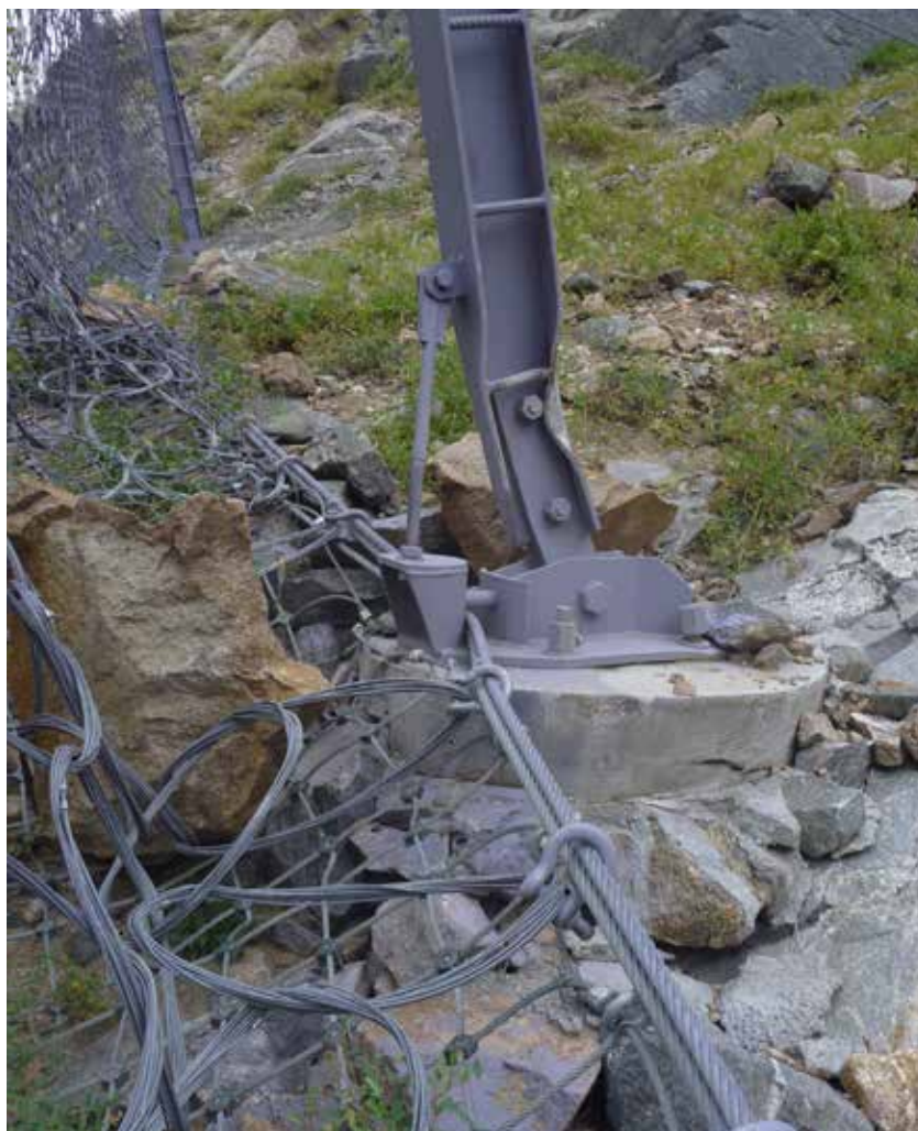
Figure 3. Rockfall barrier post supported on bedrock at Georgetown Canyon, CO, showing continued post-strike performance. (Photo courtesy of Colorado DOT.)
