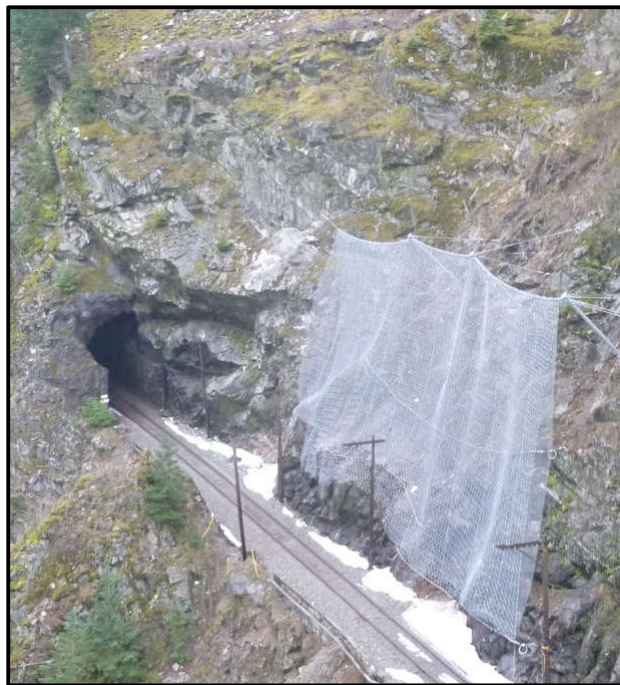
Figure 2. Typical Attenuator installation showing a series of hinged posts with support cables, and a freely hanging net.
