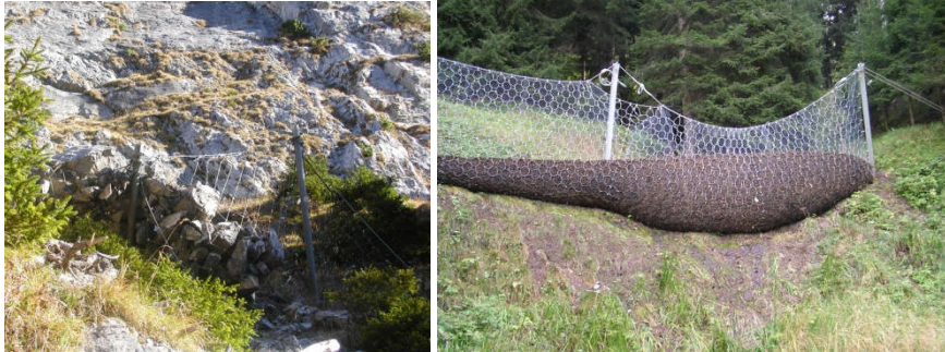
Figure 1. (left) Snow net barrier loaded with rockfall, (right) rockfall barrier loaded with a shallow landslide.
