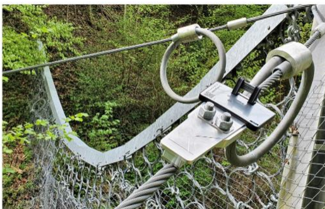
Figure 1: Geobrugg GUARD measurement device installed on a flexible ring net barrier
