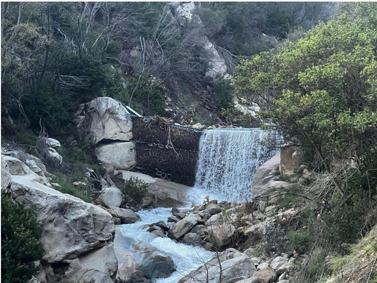
The debris net on Upper San Ysidro Creek seen Wednesday. The net is at least 25 feet high and is packed with debris after this week's storms. Pat McElroy photo
