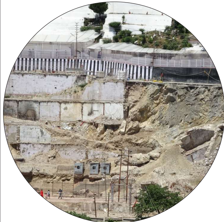
Due to heavy and continuous rain, a massive landslide occurred on the track between elevator point and gate No. 5 at Bhawan during construction of a new Bhawan at the dismantled aged Durga Bhawan.
