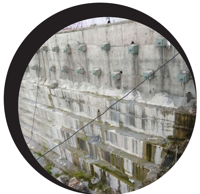
View of restored track at Durga Bhawan by construction of RCC Cladding and 100T capacity Cable Anchors
