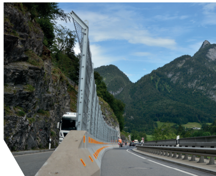
The system has proven itself on road construction sites and various race tracks worldwide.
