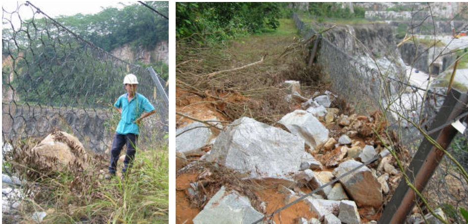
Figure 17. Barrier subjected to combination loads, detachment of single blocks and shallow landslides with granular material.
