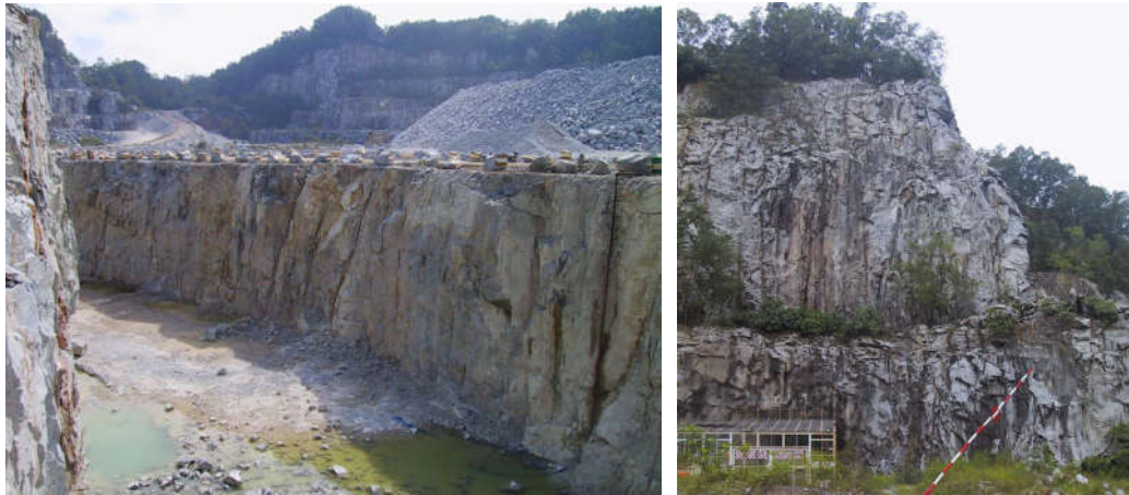
Figure 13. Inner and outer trench walls from CH 490 to CH 1100 (left) and walls + slope above lower bench from CH 1600 to CH 1650 (right)
