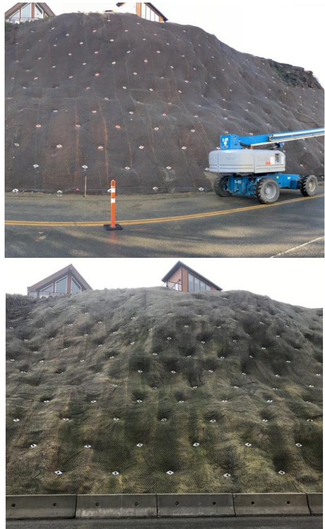
Figure 10. Condition of the slope in October 2016 (upper) and in February 2017 (lower) – in the process of revegetation 4 months later.
