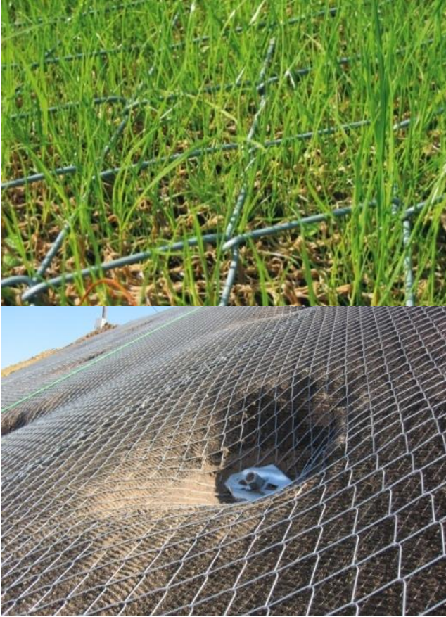
Figure 2. High-tensile wire mesh (upper) and spike plate to tension the high-tensile steel wire mesh against the slope surface (lower).
