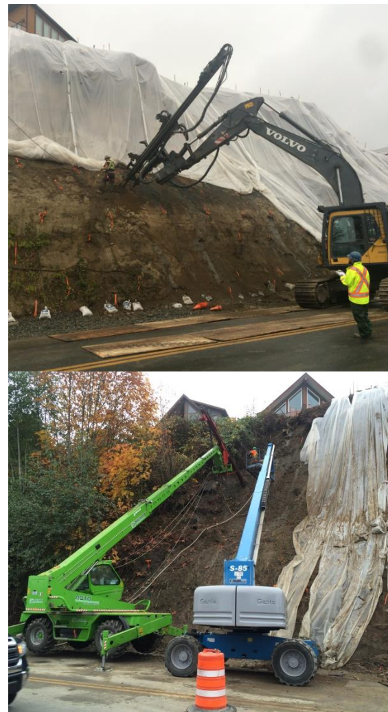
Figure 9. Installation of soil nails with excavator (upper) and zoom boom beside a man-lift (lower).
