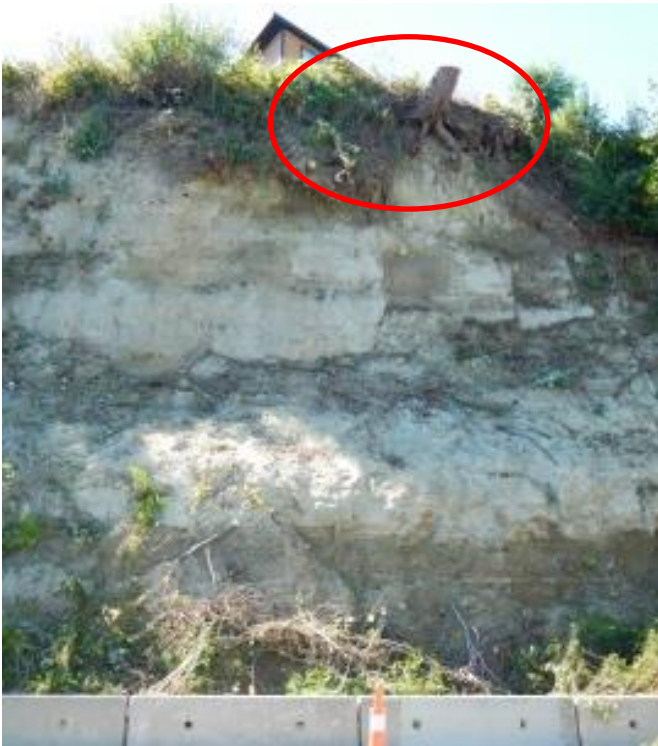
Figure 8. Roots and loose granular soils at the crest.
