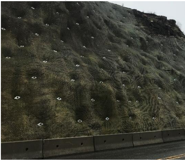
Figure 4. General profile with the nail arrangement (upper) and staggered pattern of nail installations at Cowichan Bay Road (lower).
