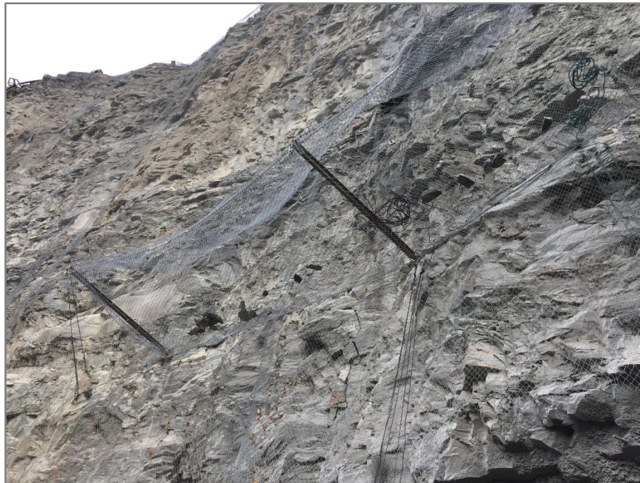
Figure 6 – Adit canopy rock debris subject to maintenance cleaning (Photo by Scarpotec, Inc.)
