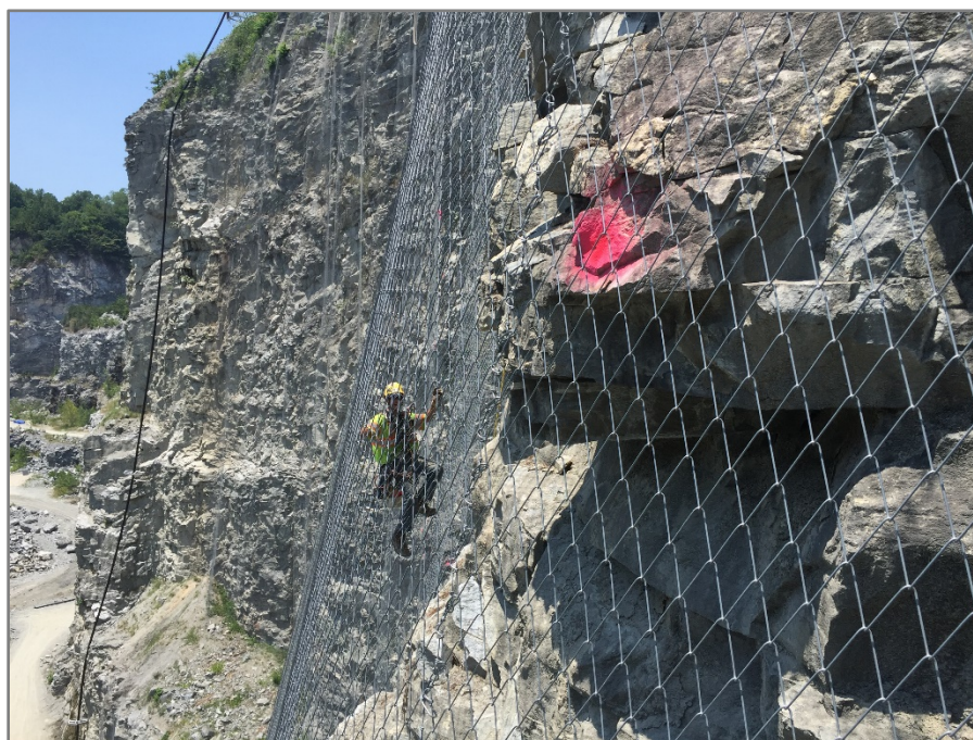
Figure 3 – Rock dowel layout with paint using rope access (Photo by Scarptec, Inc.)
