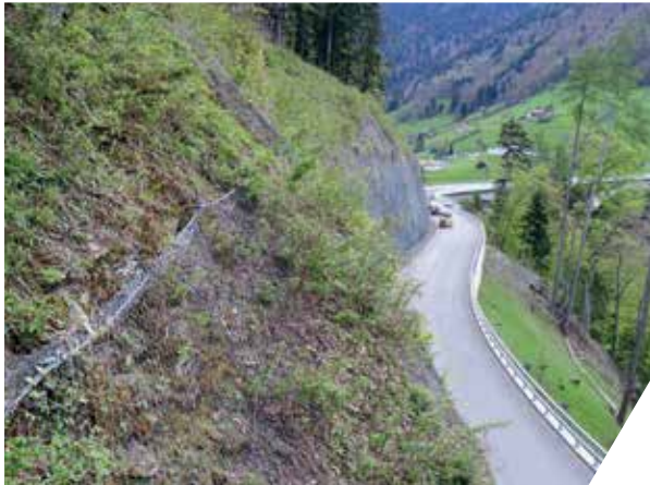
Rockfall Drapes (Anchorage of Support Rope)
