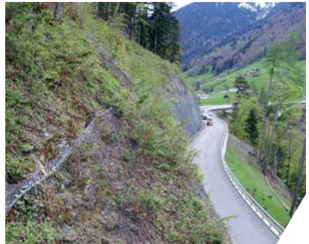
Rockfall Drapes (Anchorage of Support Rope)
