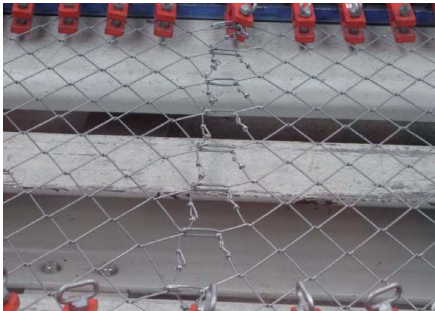
Condition right before the collapse of the mesh
