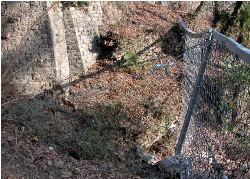
Fig. 7: Side view of barrier no. 3 (UX), located upstream from the bridge on Barcone Street
