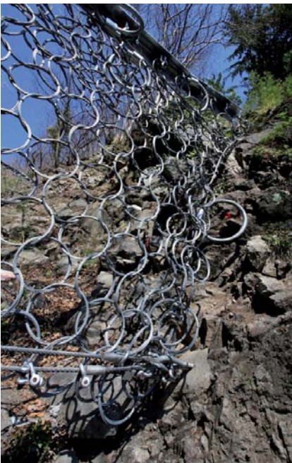
Fig. 3 (above): Detail of barrier 3 (UX) on the left bank of the torrent
