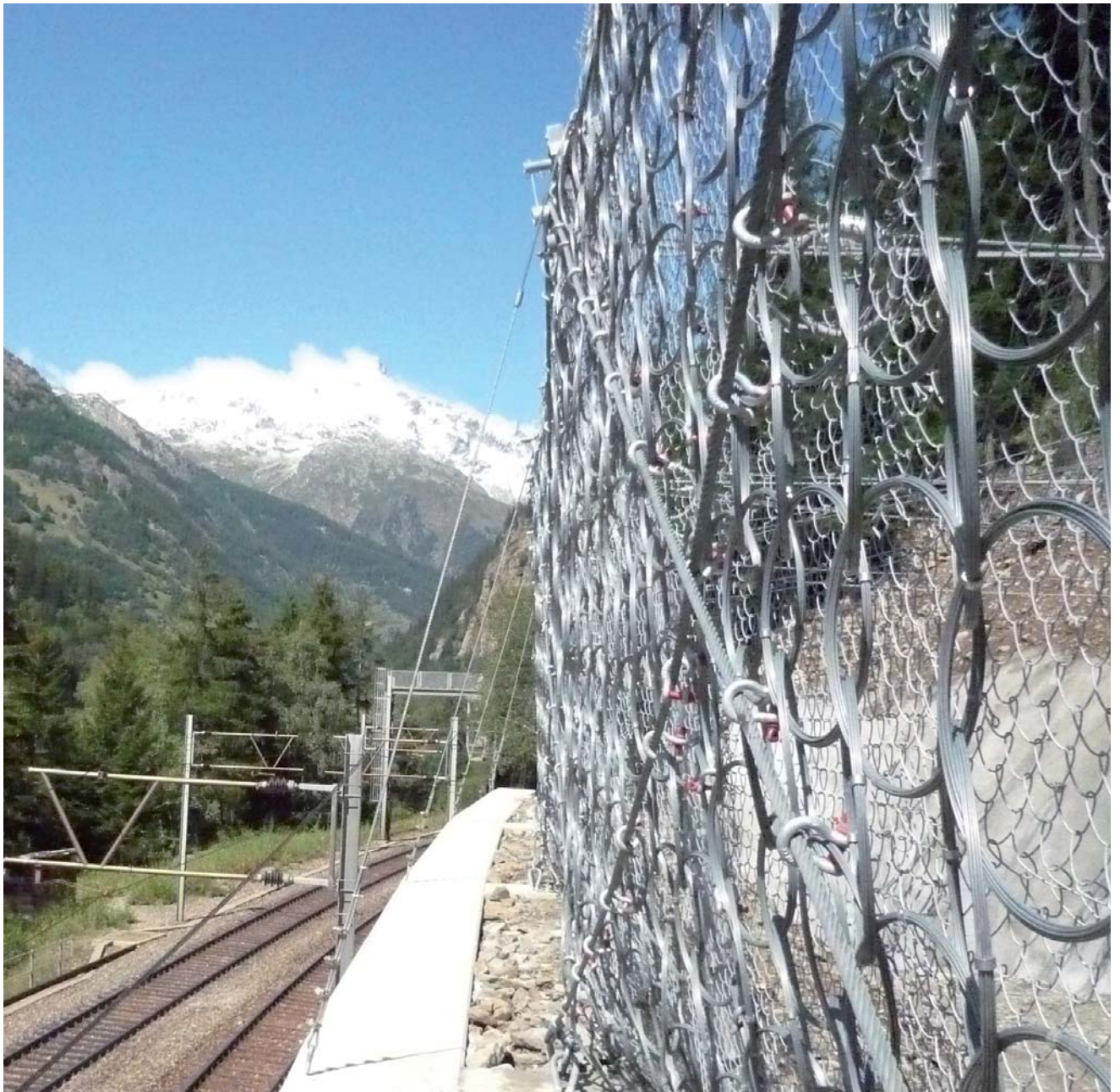
Low-deflection barrier "Bubichopf gallery" BLS Goppenstein–Brig line / Switzerland
