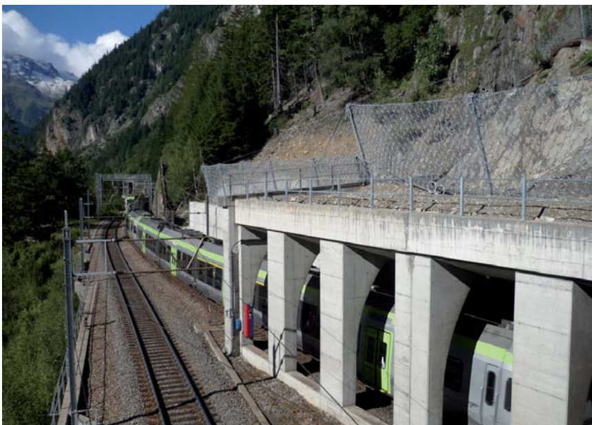
The RXI-100 rockfall protection barrier serves both to protect the gallery and to extend it to protect the rail line
