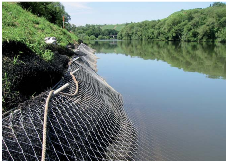
Submerged TECCO® mesh below the water level
