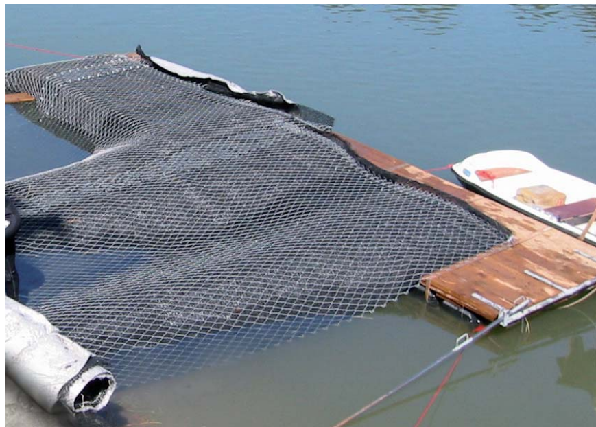
Preparing the TECCO® mesh for placing under water with a mobile raft
