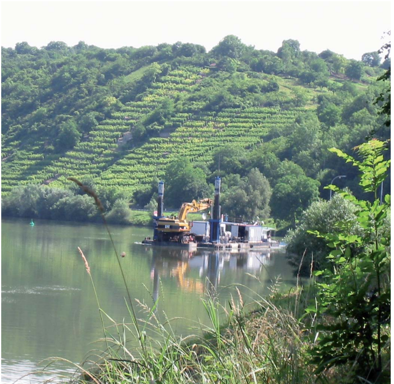
Repairs to a reach dam using TECCO® steel wire mesh and pillar Neckar Federal Waterway, fall at Besigheim / Germany
