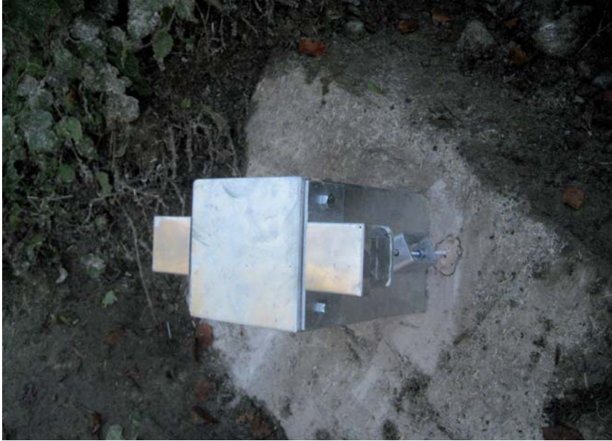
Installed ABOXX with special geometry
