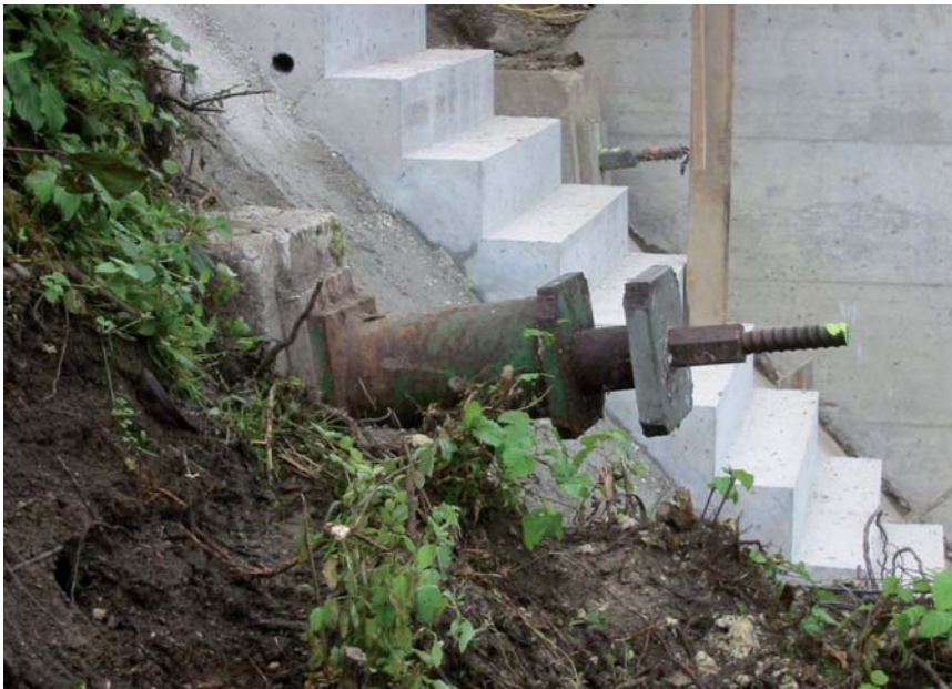
Corroded post tensioned anchor prior to the ABOXX installation
