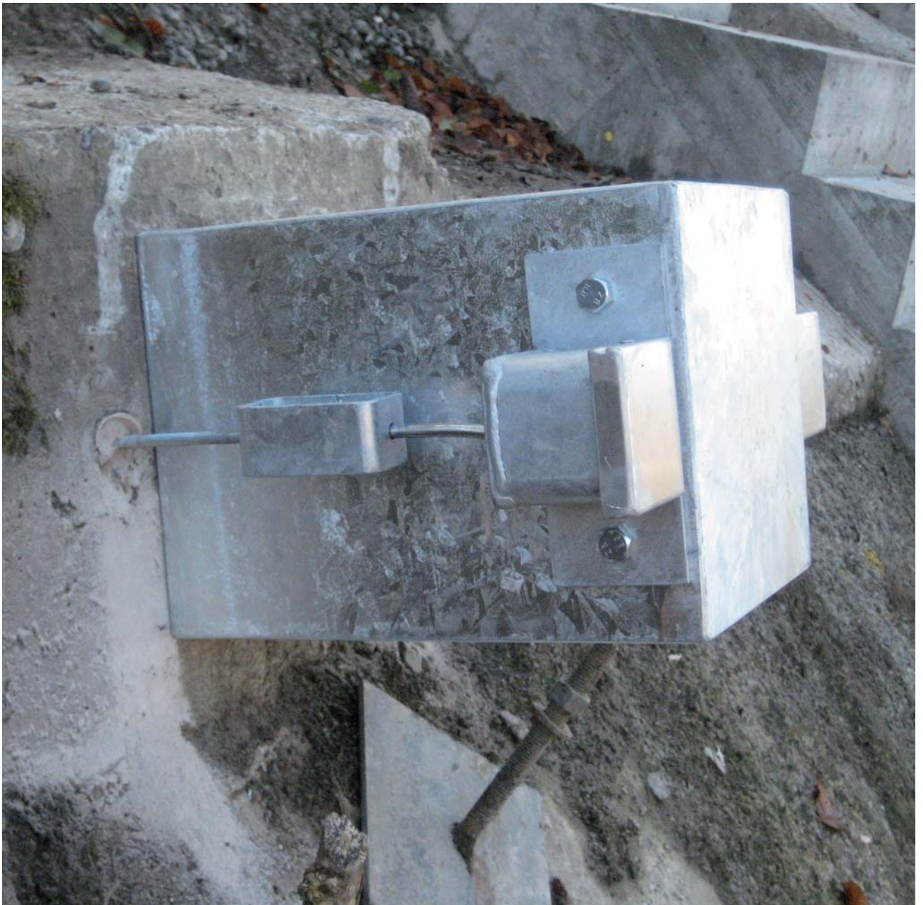
Anchor protection Rosenberg (Freeway A1), St. Gallen / Switzerland
