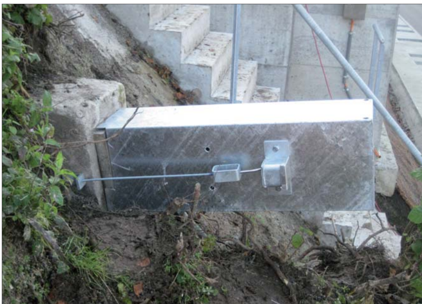
Corroded post tensioned anchor protected by means of an extra length ABOXX
