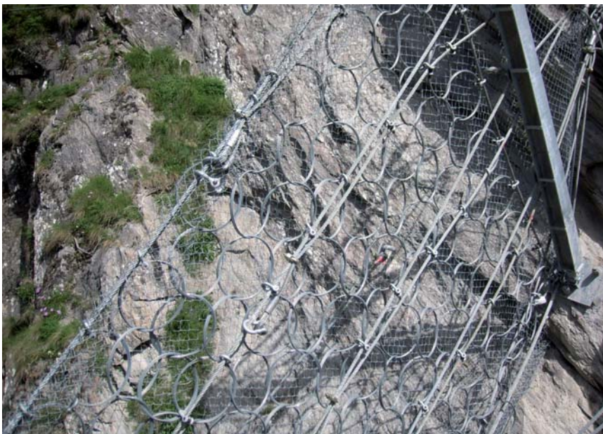
Deflector protection with three central, one upper and one lower suspension cable incl. running ropes in the post areas. The posts were specially developed for this project.
