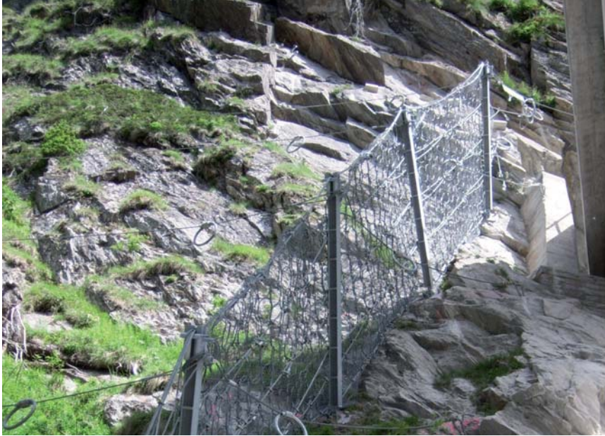
Employing long retaining ropes enables the anchors to be relocated out of the danger zone.
